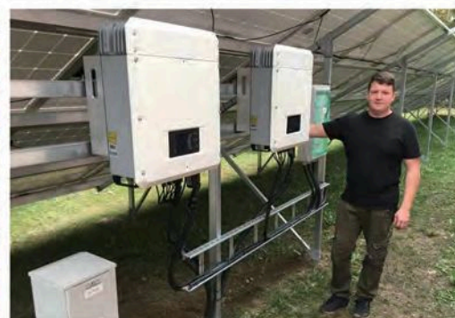
Photovoltaic inverters in European photovoltaic parks project
