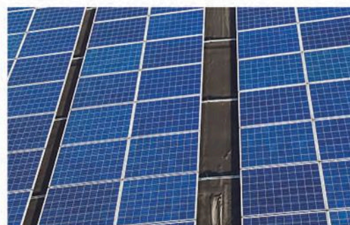
Distributed project of Dahai Group factory
