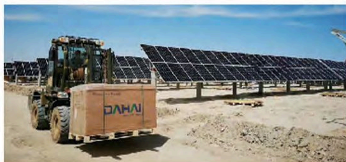
Laiwu Jinneng power station project 13MW
